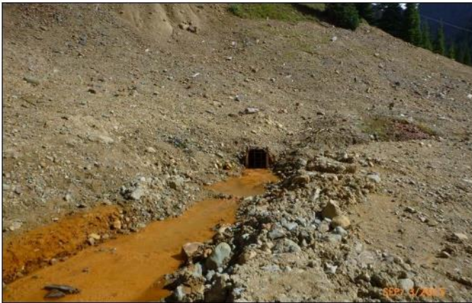
Figure 7.—Photograph showing the seepage outflow from the drain pipe at the American Tunnel at Gladstone, Colorado, as it appeared on September 3, 2015, with about 100 gpm of acid water flowing out.
