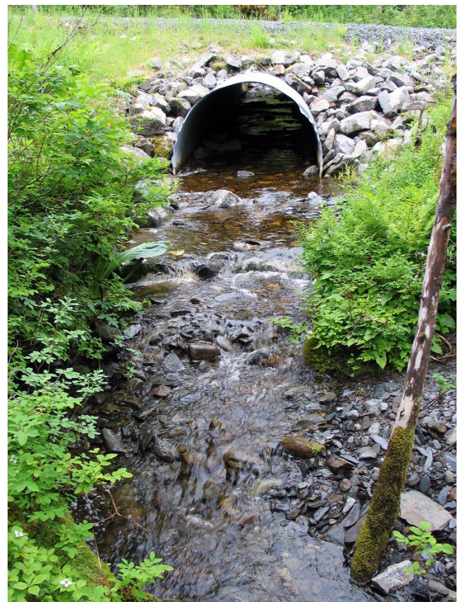
Perched and velocity barrier culvert replaced with a Stream Simulation designed 78" x 36ft long round corrugated metal pipe. Note: This pipe survived a greater than Q50 (2% Annual Exceedance Probability) event with no maintenance required. Tongass NF. Credit: Bob Gubernick, USDA Forest Service.
